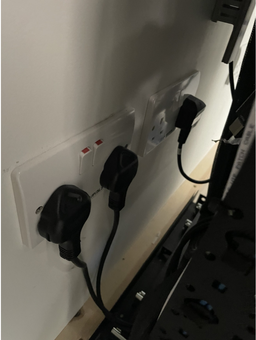
BT Network Switch and Loudspeaker control box power at rear of of rack
